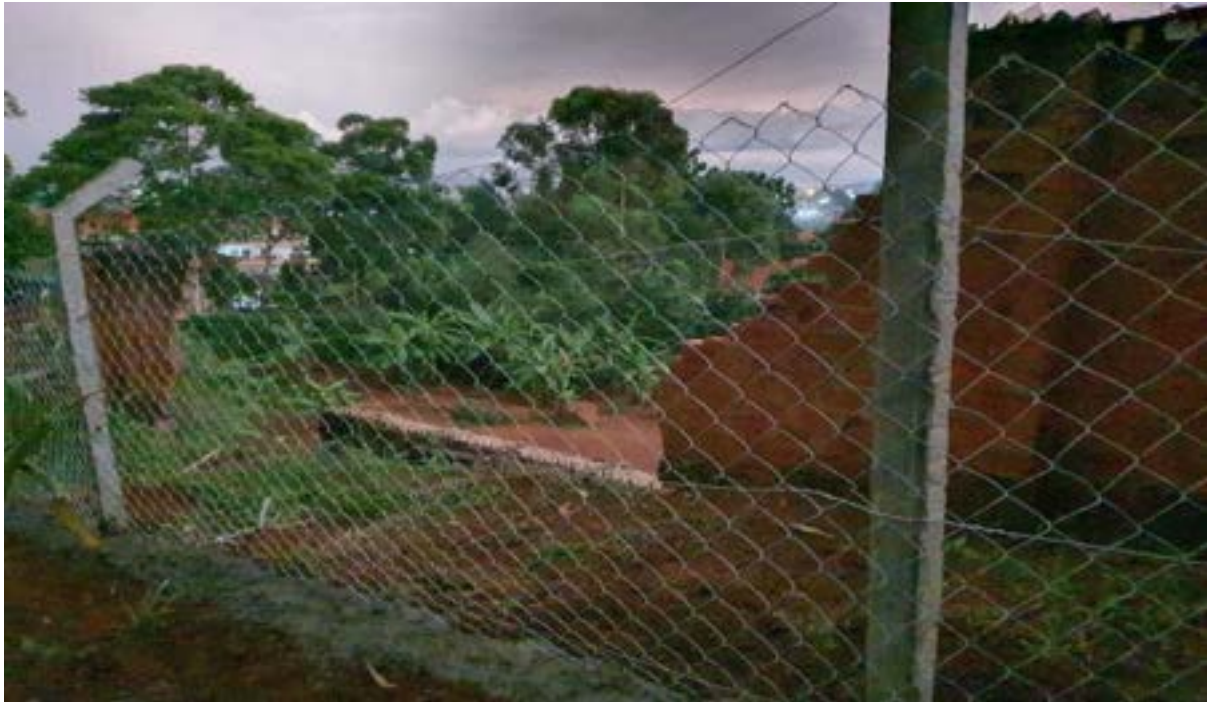
The broken part of the perimeter wall and the temporary chain-link fence
